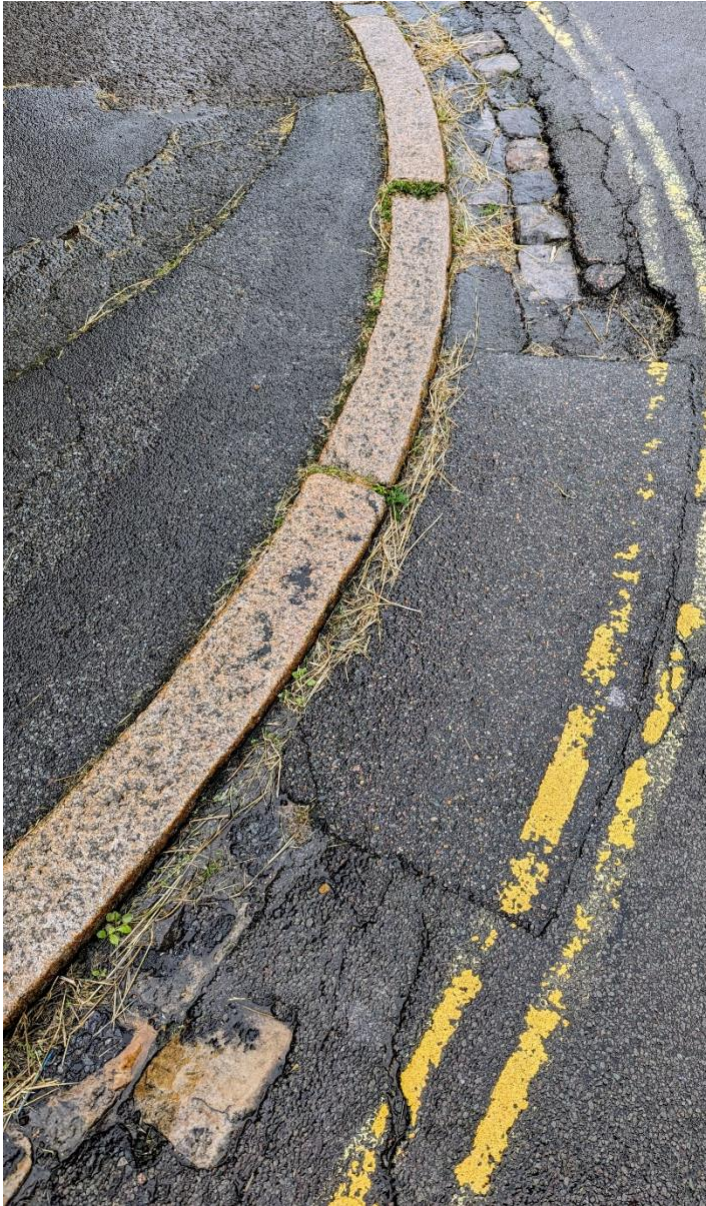
Example of granite setts unnecessarily covered by bituminous macadam within the conservation area at Valance Road.
